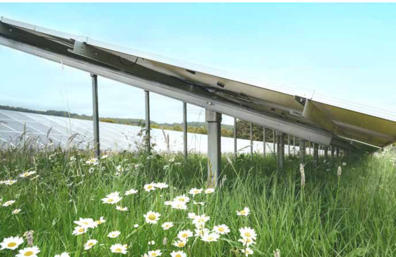
A solar mounting structure by MEISER Solar in Morscholz
