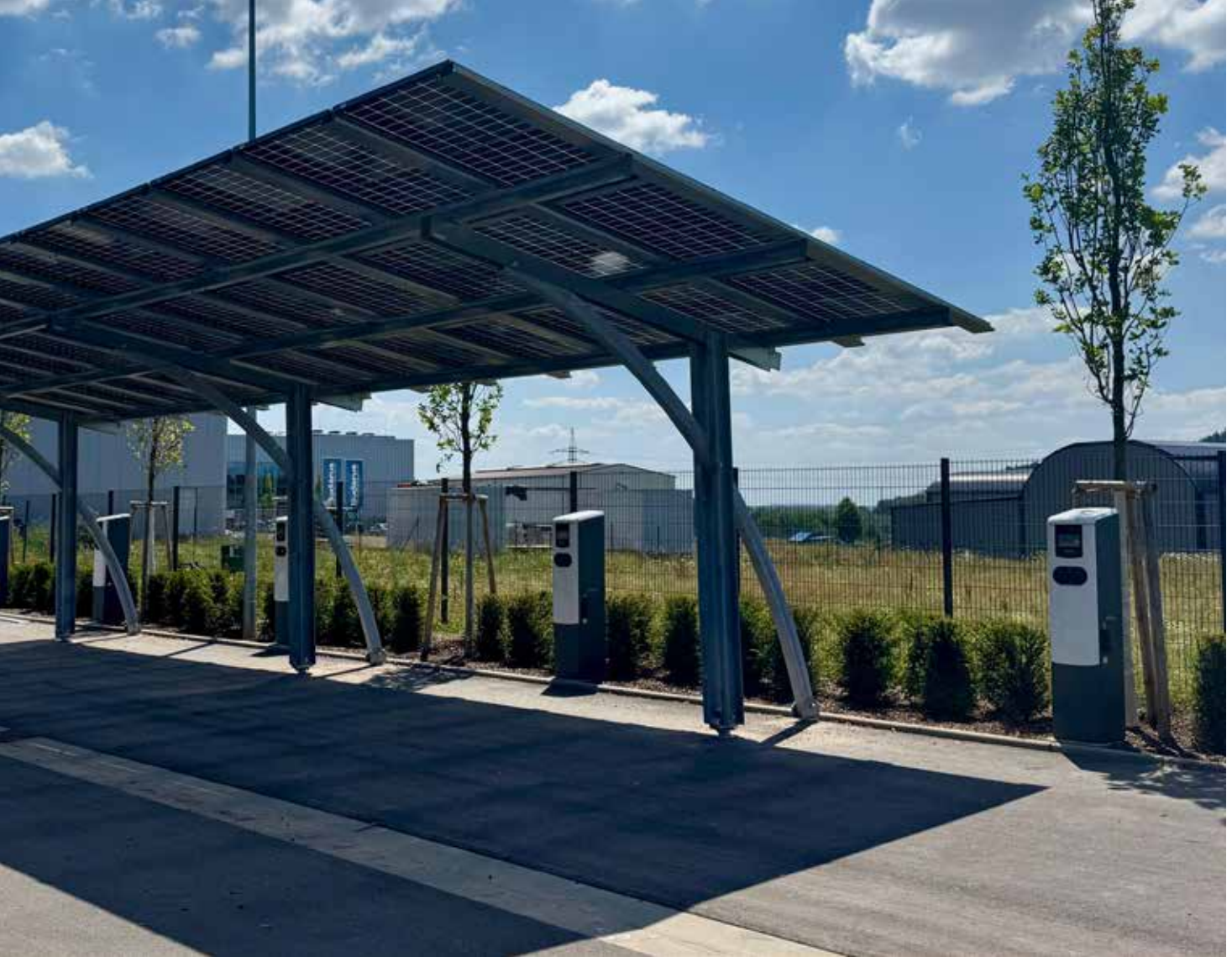
VOLTWING ECO on the MEISER site in Losheim am See
